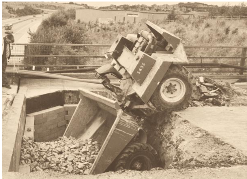
Figure 14 Small site dumper fallen into excavation due to lack of wheel stops
